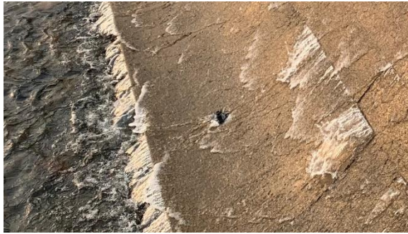
Photo 16A: Photo of BH113 at the south side of the spillway, note the tubes for the piezometers sticking out from the borehole
