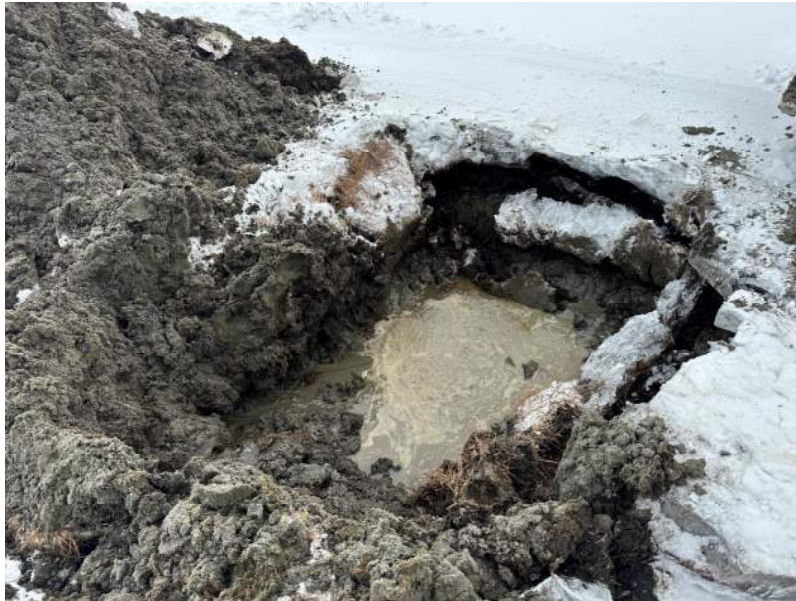
Photograph 11 Water accumulation in TP20.
