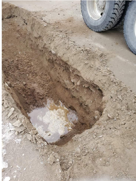
Photograph 9 – September 22, 2021 Groundwater seepage in TP06.
