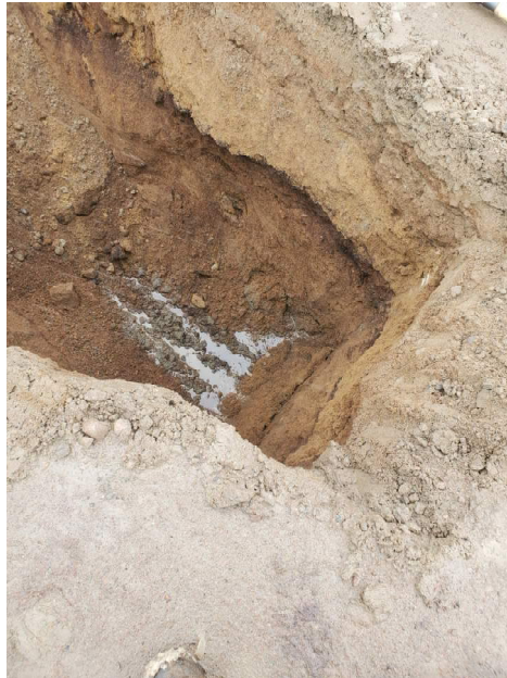
Photograph 7 – September 22, 2021 Groundwater seepage in TP05.
