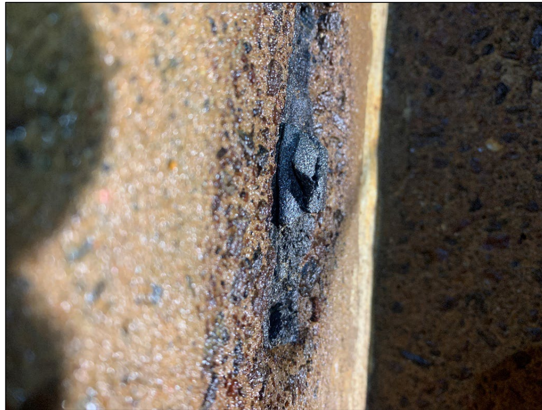
Close-up of black tar-like substance
